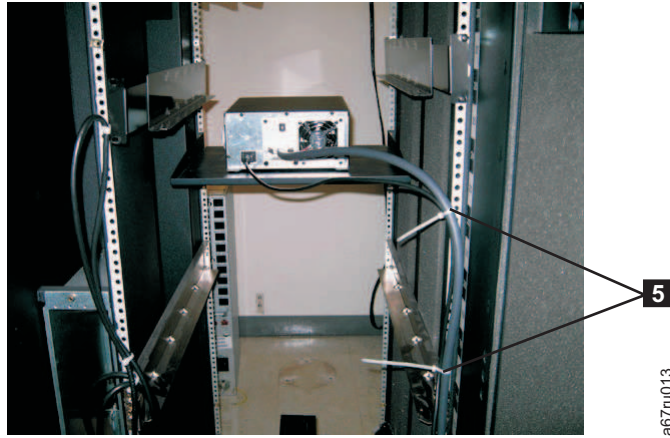
Figure 30. Rear view of shelf with cables attached to rack rails with tie wraps
